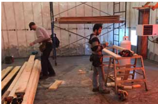
Work continues on schedule for water installation to the new White Sands Truck Fill station which is scheduled for completion this spring.
