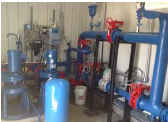
A glimpse at the waterworks inside the Big Valley Truck Fill which County employees from our Environmental Services Department monitor and maintain.
