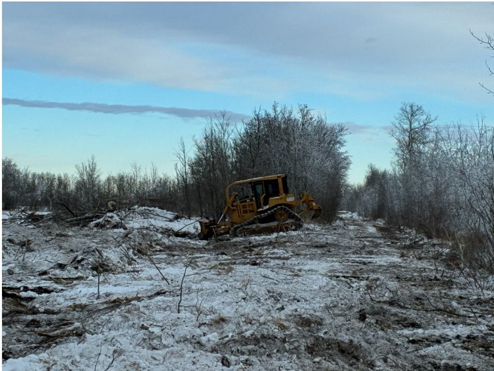
PW Figure 0.12. North Of Warden On Rge Rd 20-2 - Dozer Doing Fenceline Brushing
